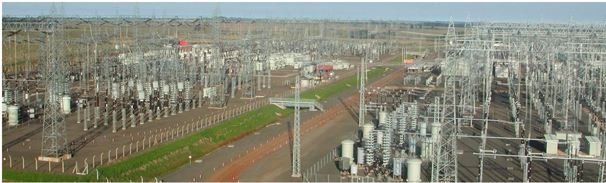
The Garabi high-voltage direct current converter station
